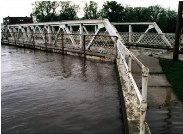
Volga Bridge Washed Away in Flood Event
