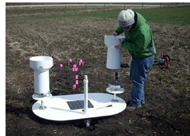
Rain Gauge Installation in the TRW
