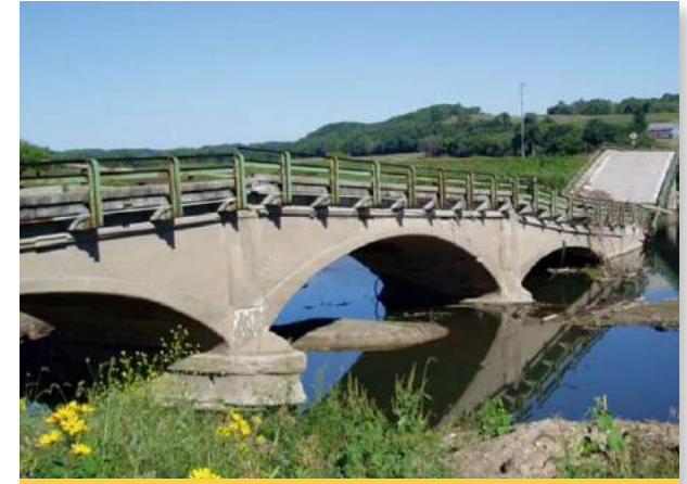
Fayette County Bridge Damaged in Flood Event
