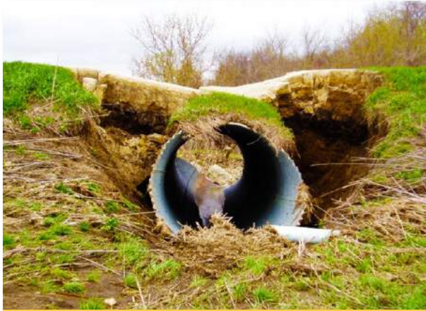
County Road Infrastructure Damage
