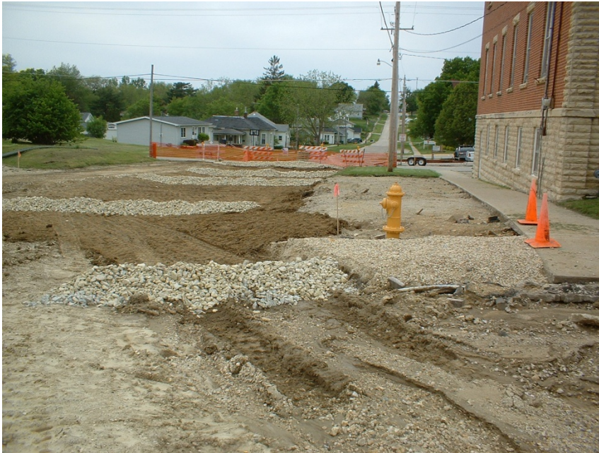
Crushed Stone Check Dams
